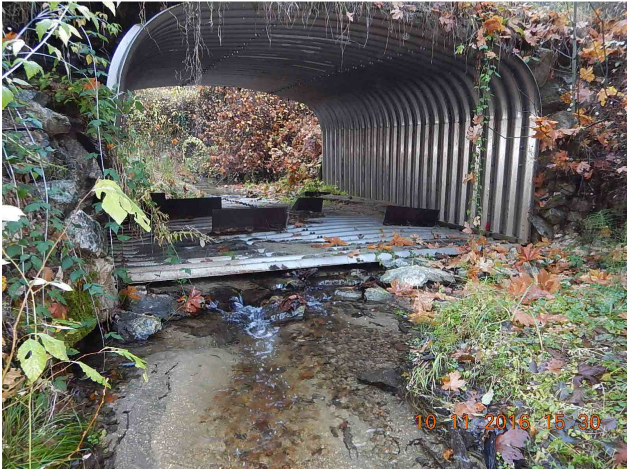
Figure 10. Barrier #3 - The decommissioned BLM road culvert is passable either by burst-attach swimming through the flat-bottomed culvert or, more probably, by crawling underneath. The stream has fully excavated under the culvert bottom, providing unimpeded passage.
