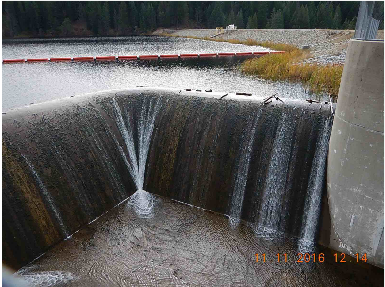
Figure 19. Buckhorn Spillway - Section E: The upper spillway wall (height 20 ft, with a slight incline; photo at reservoir elevation 2803.00 ft).
