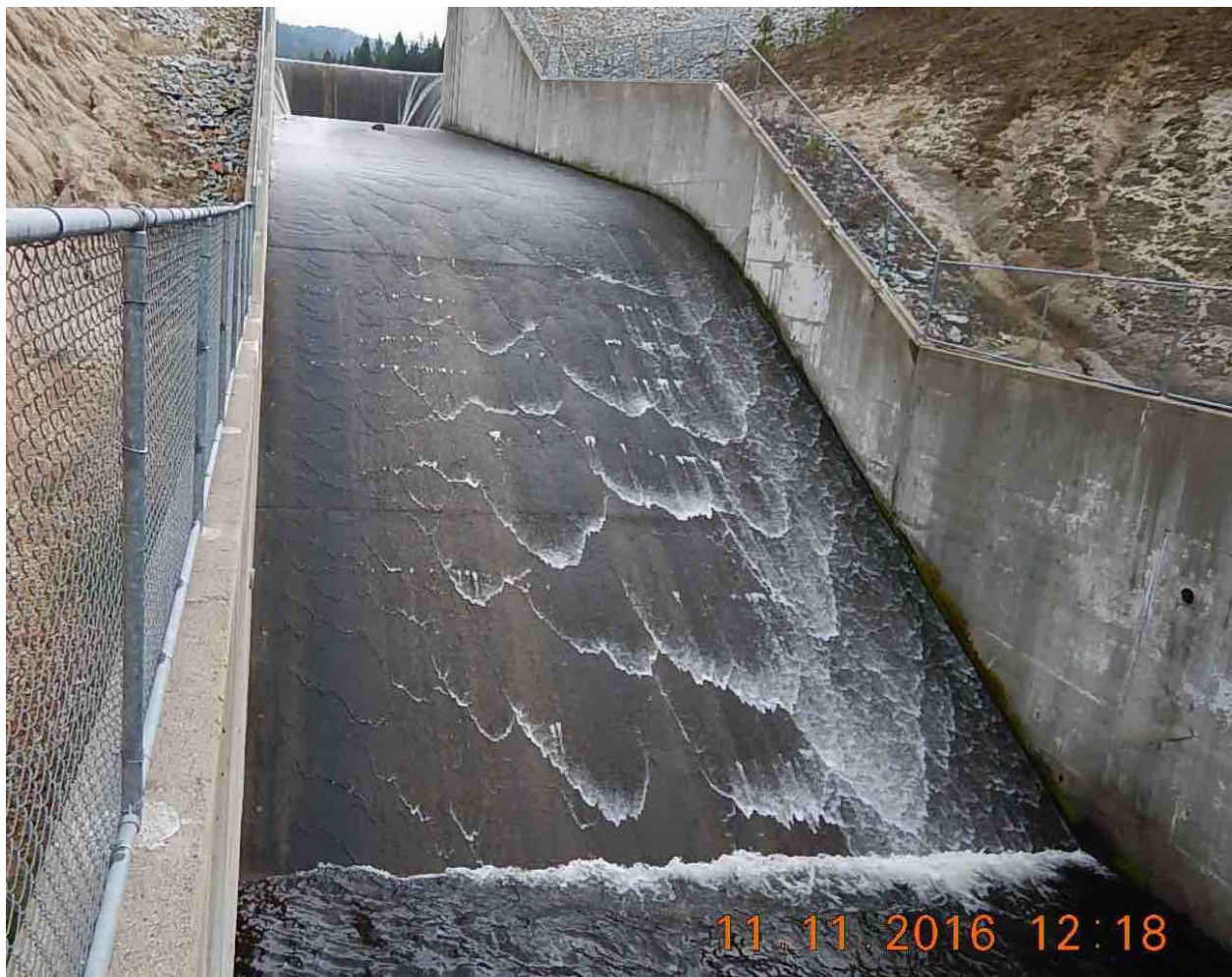
Figure 18. Buckhorn Spillway - Section D: The upper ramp (length 275 ft, \sim 10^\circ - 45^\circ ).
