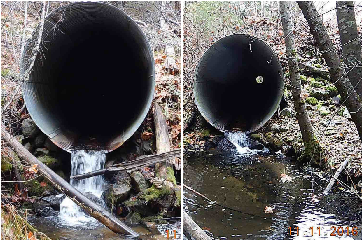
Figure 12. Barriers #5 a, b - Highway 299 "double-crossing" culverts below Buckhorn Summit. A) entry to lower culvert, B) entry to upper culvert.
