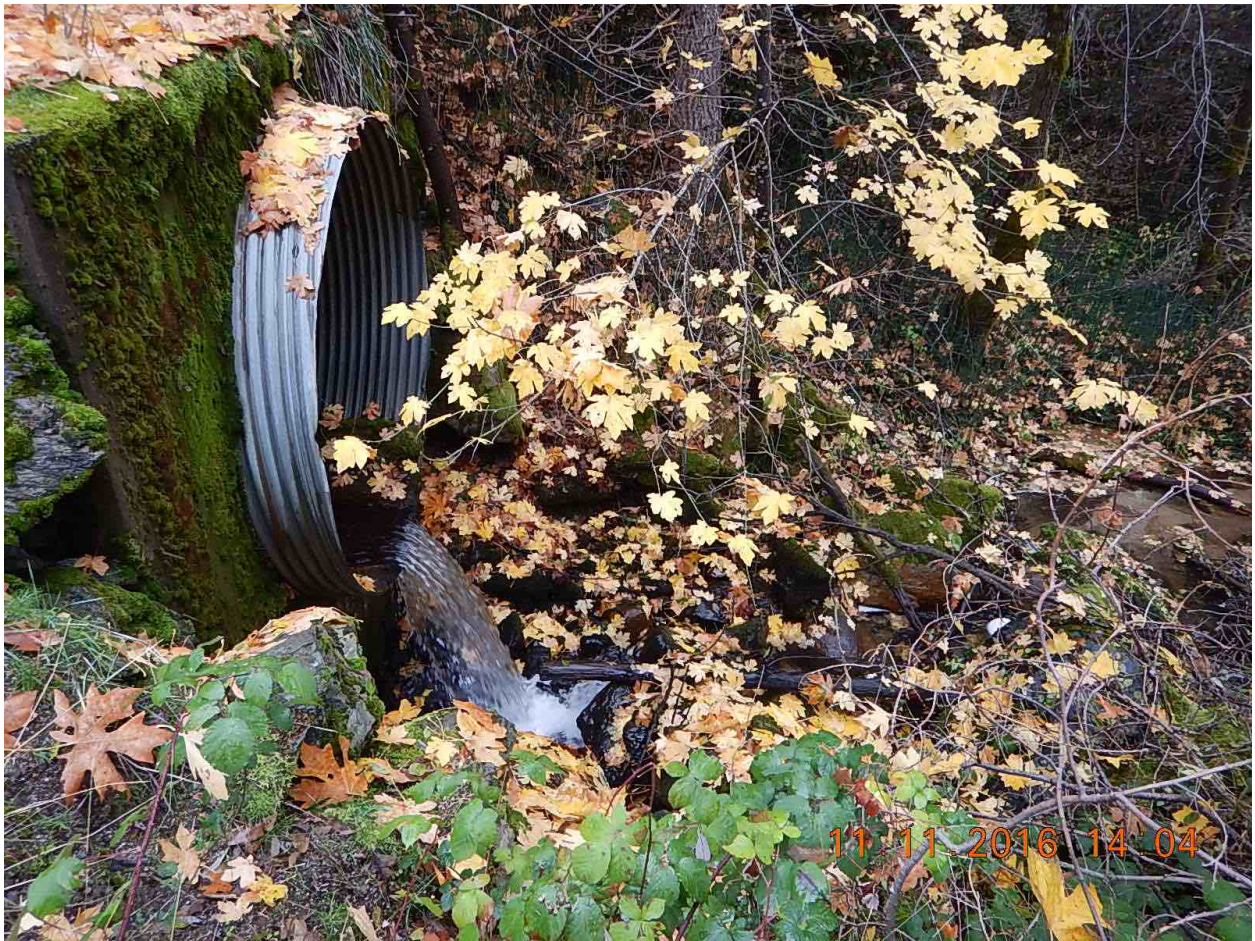
Figure 11. Barrier #4 - Private entry (TriL Ranch), a perched culvert (5 ft drop) with an overhanging edge and impassable.
