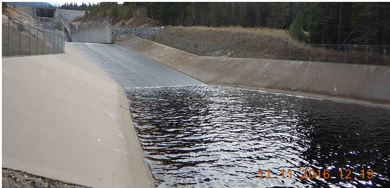
Figure 17. Buckhorn Spillway - Sections A and B: Entry pool and lower ramp (ramp length 180 ft, ~ 8° incline).
