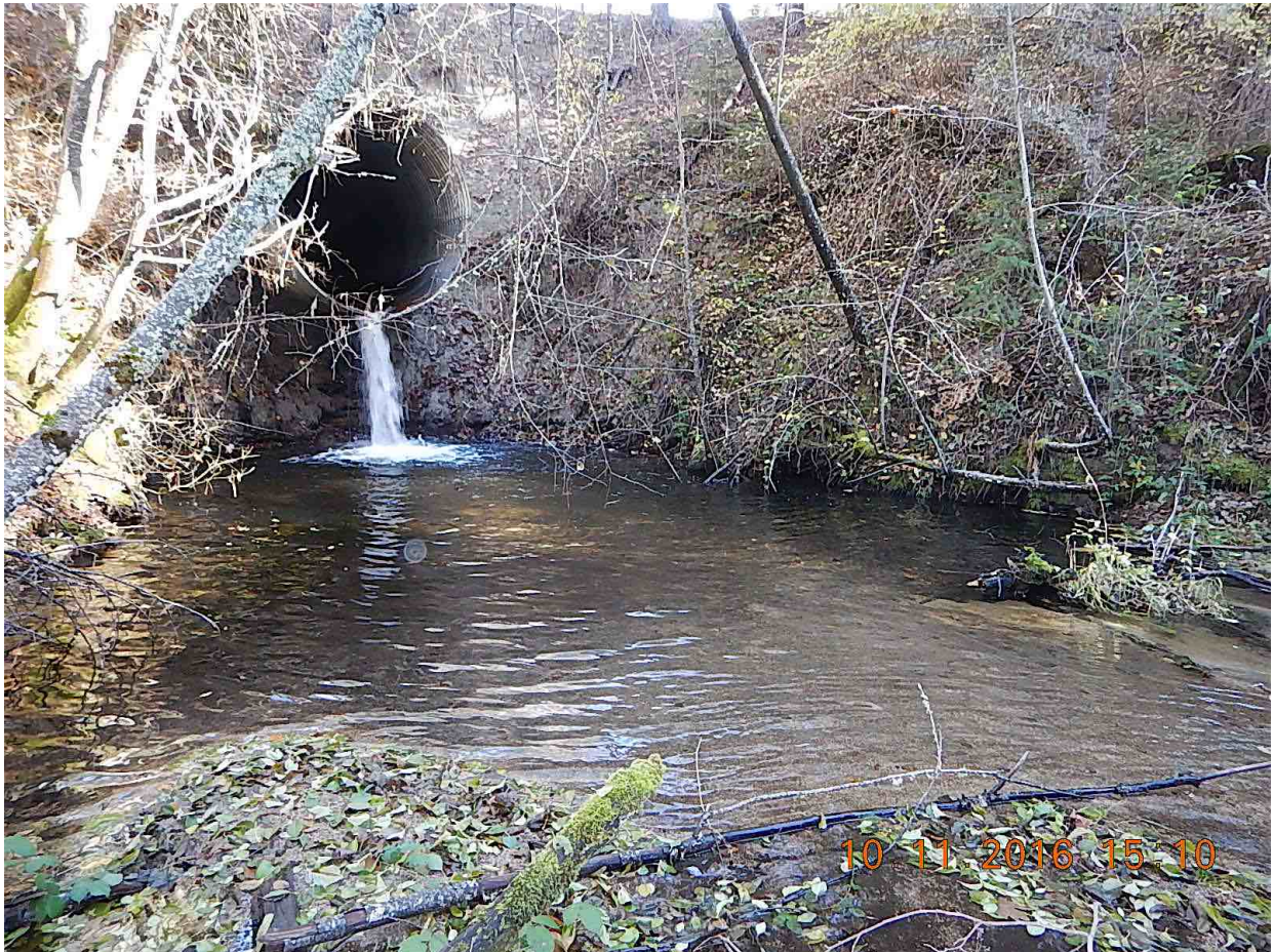
Figure 8. Barrier #1 (Little Grass Valley Creek, see map) - I.O.O.F. entry on lower Little Grass Valley Creek. This is a large perched culvert (5 ft drop) that blocks the drainage, 600m upstream of the confluence with Grass Valley mainstem.
