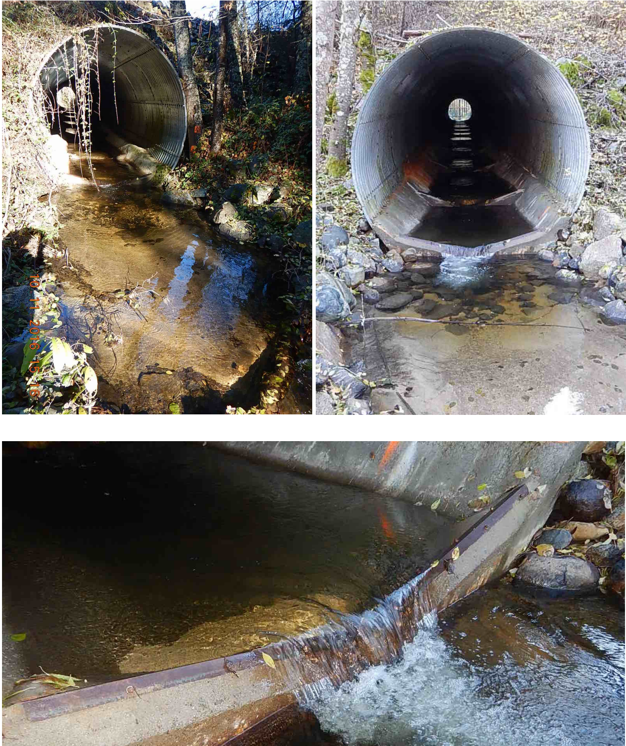
Figure 9. Barriers #2 a,b - Highway 299 culverts at Buckhorn Station. A) entry to lower culvert, B) entry to upper culvert, C) interior baffle design.
