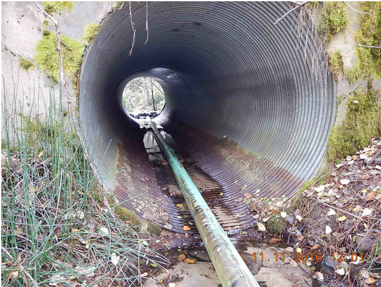
Figure 13. Barrier #6 - Shingle Shanty crossing, Buckhorn Dam road. The relatively short culvert represents a minor passage impediment due some increased effort to pass at higher velocities. It would not particularly benefit by modification, other than replacement with a fully natural bottom.
