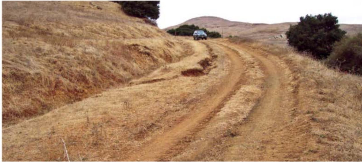
FIGURE 224A. Ditched, gullied, deeply rutted, and bermed seasonal road before being converted to an outsloped road with rolling dips.
