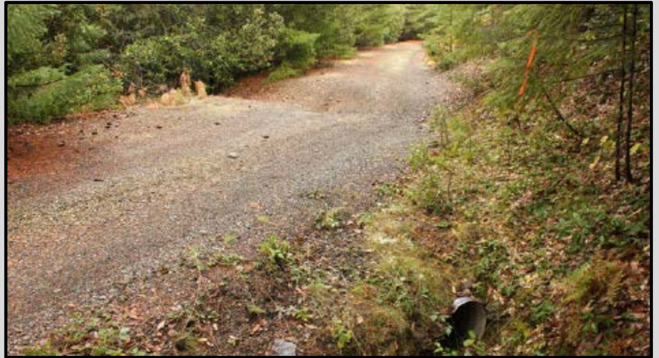
Figure 4- An Example of a Waterbar and Ditch Relief Culvert used in Concert (Weaver et. al 2005).
