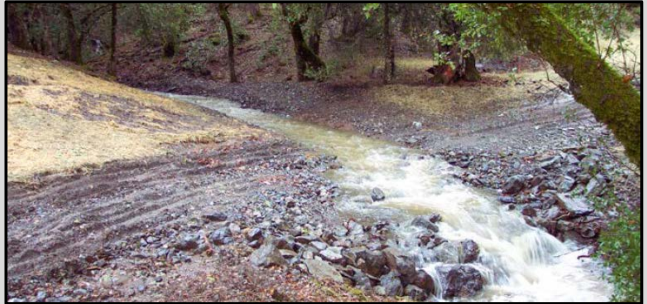
Figure 3- A Properly Constructed Stream Crossing on a Seasonal Road (Weaver et. al 2005).
