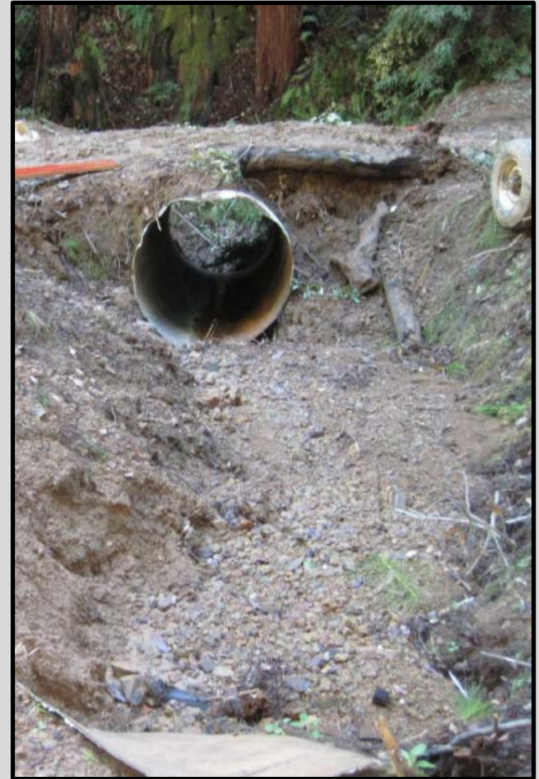
Figure 2- An Image of a Non-Compliant Culvert (Manthorne N.d.).
