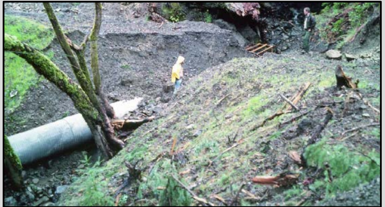
Figure 18- An Example of the Potential Results of Neglecting Culverts (Weaver et. al 2015).
