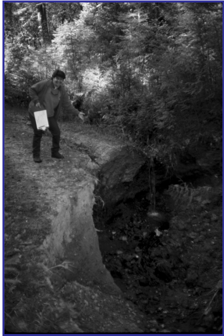
Road problem discovered during inventory
