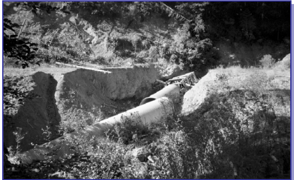
Failed culverts are a common road-related problem
