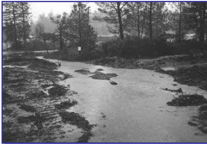
An erosion problem at a construction project
