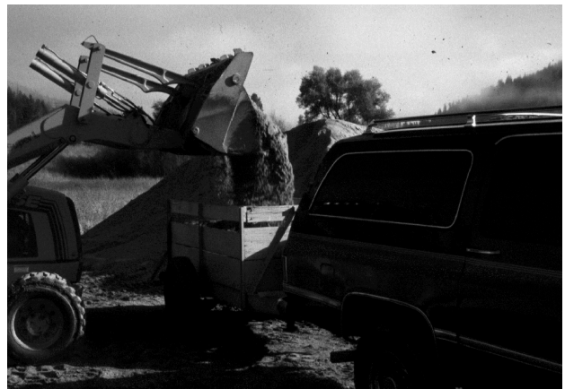
Load 'em Up: Loading a Trailer with Free Sand at the Give-Away Day.
