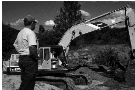
Project Manager John Condon Supervising the Dredging Operation at the Hamilton Ponds
