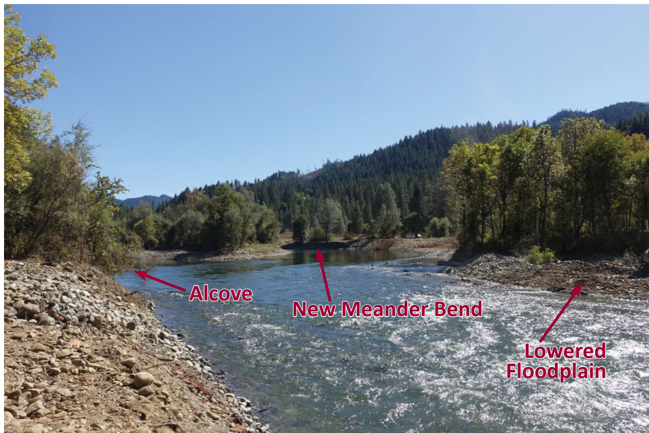
Newly constructed meander bend (top right) and alcove (top left), upstream of a gravel bar and lowered floodplain (right)
