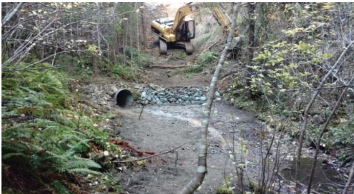
Inlet basin cleaned and rip rap placed at inlet of existing culvert.
