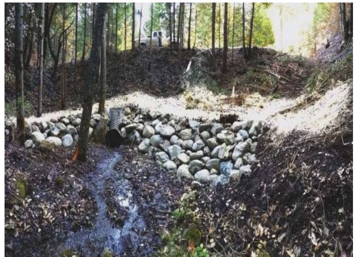
Inlet basin cleaned, rip rap placed at inlet and saddle riser added to existing culvert.
