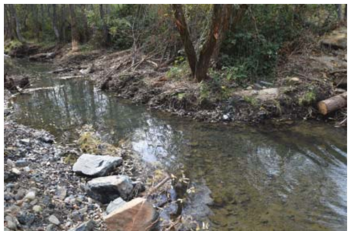
Constructed low flow side channel provides rearing habitat for juvenile salmon and steelhead.
