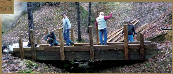
Installation of handrails by TCRC D employees (l-r) Jeff McGrew, Duke Klang, John Condon and Darrel Tate. Doug Crispin works on underside of bridge.
