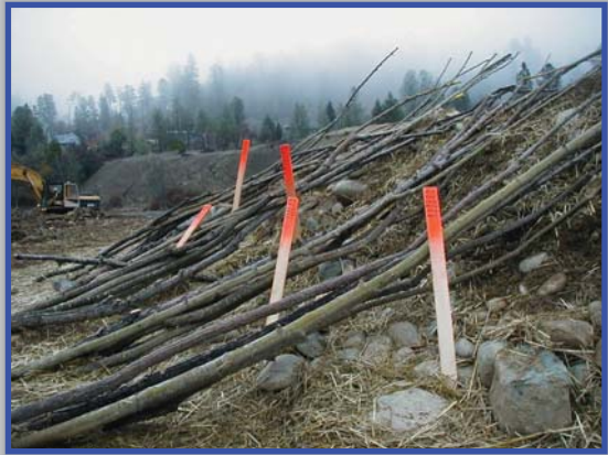
Cuttings ready for mechanical cluster planting to ensure they reach the water table.
